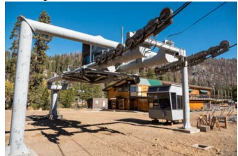
New quad Chair #6 set to carry 60% more skiers and boarders to the slopes this season. ing just outside the main Day Lodge and bringing skiers and riders just under 3,000 feet in distance and 800 feet in vertical rise.
